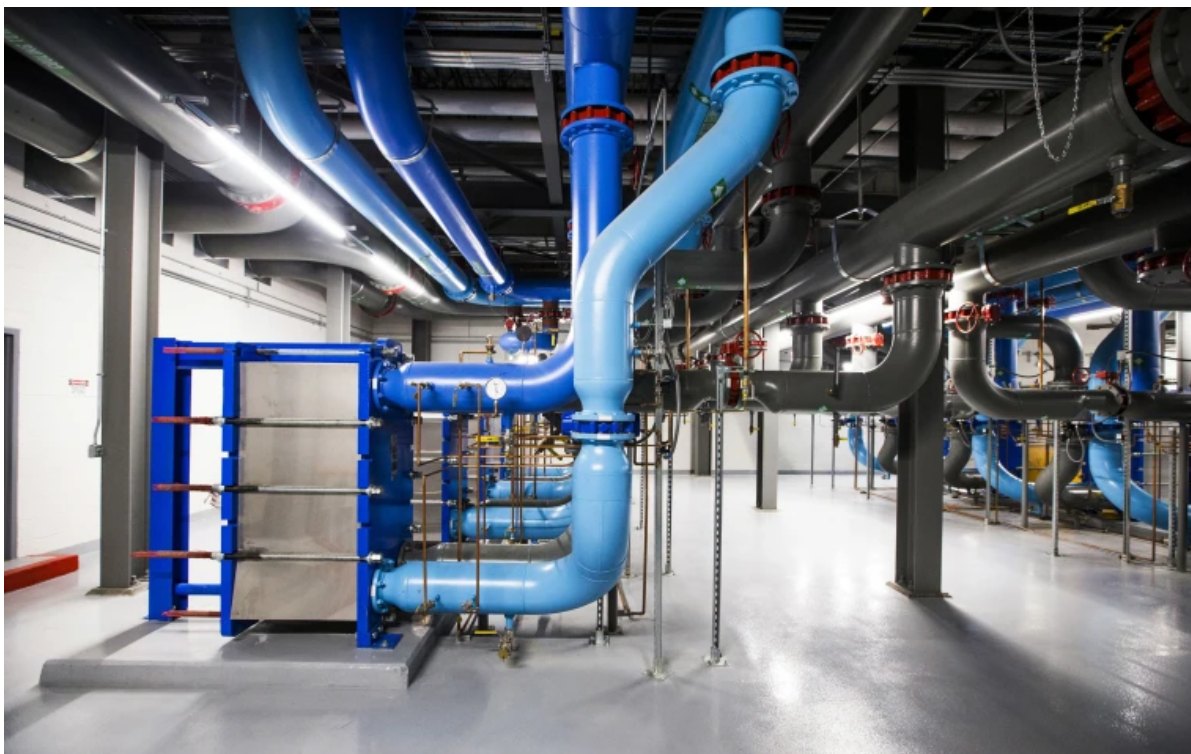
The system used to cool servers inside the Apple Data Center in Mesa, Ariz. Tom Tingle / The Republic / USA Today Network
